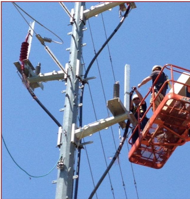
KCS technicians assembling the final Tyco Heat Shrink Termination on the 60' riser pole.
