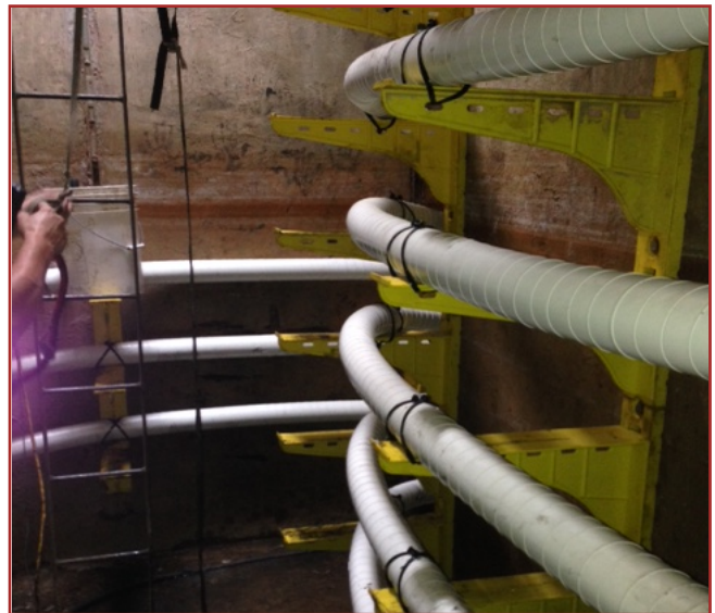
View of the new installation of Kerite's 138kV system wrapped with arc flash tape.
