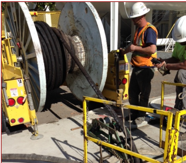
Removal of the vintage 1950's low pressure oil filled cable with the use of a 20 ton puller.
