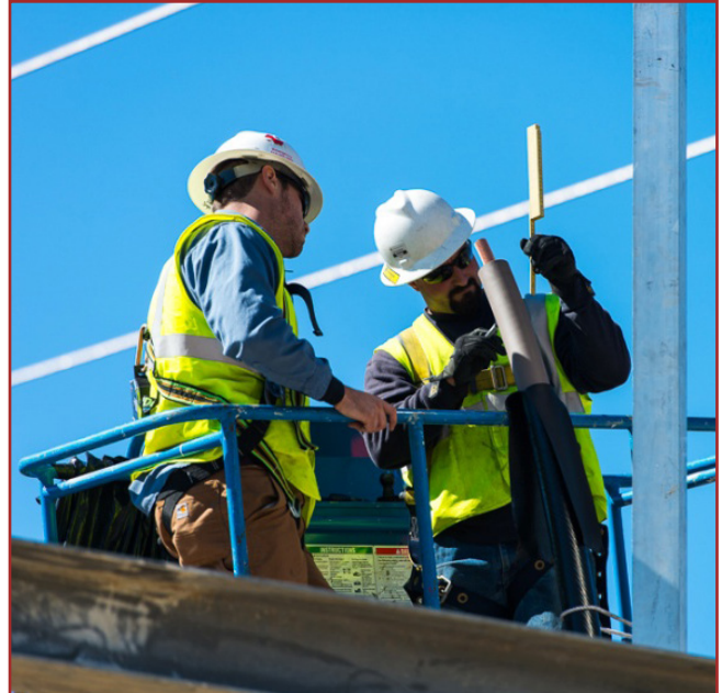
KCS technicians prep cable for terminal connector.
