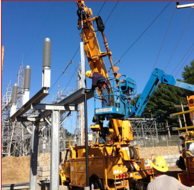
Pulling the cable up the riser structure and securing to a cable stand.
