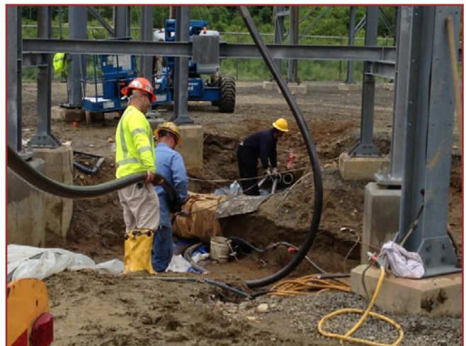
KCS's subcontractor manipulating the cable in order to secure to riser structure.
