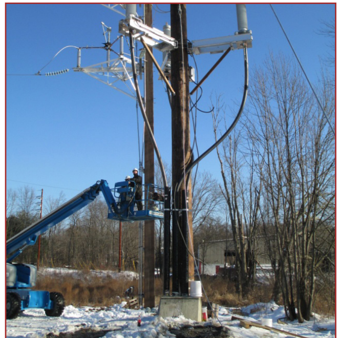
3- G&W PAT 140 installed on Riser Pole
