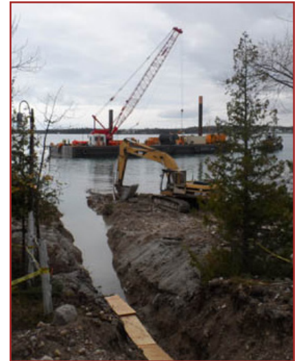
Kerite used a local subcontractor to dig trenches and install the cable
